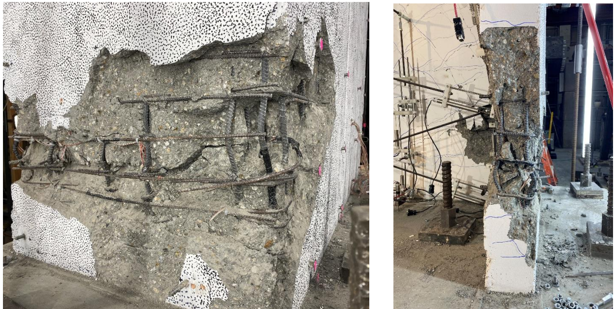
Figure 4-6: West flange close-up pictures after the test
