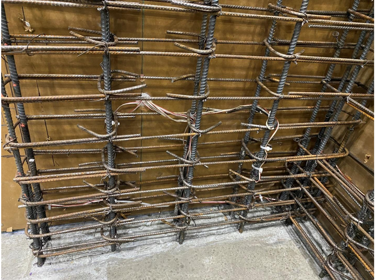
Figure D-5: CW-1 Flange reinforcement close-up
