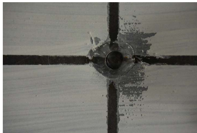
Figure 4-36. Weld fracture of tie bar at 3 rd row and 1 st column from West side of North Web.
