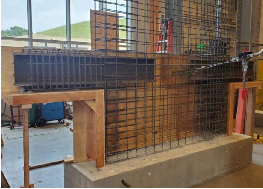
Figure 3.8. Photo of Reinforcement in Wall and Coupling Beams for SRC-W3 (right) and SRC-W4 (left)
