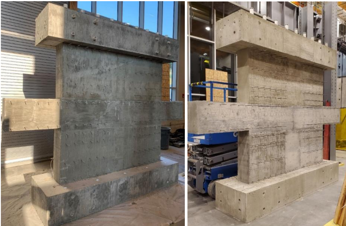
Figure 3.11. Photos of Test Specimens after Completion of Construction (Left Photo: SRC-W1 and SRC-W2. Right Photo: SRC-W3 and SRC-W4.)
