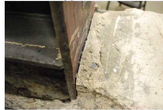
(d) Gap opening between flange and wall
