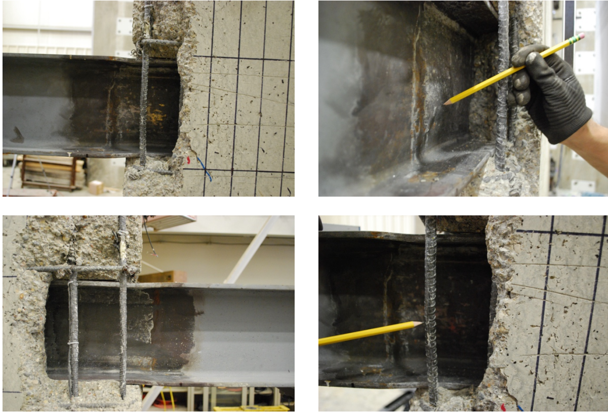
(a) Flange bending and extent of damage
