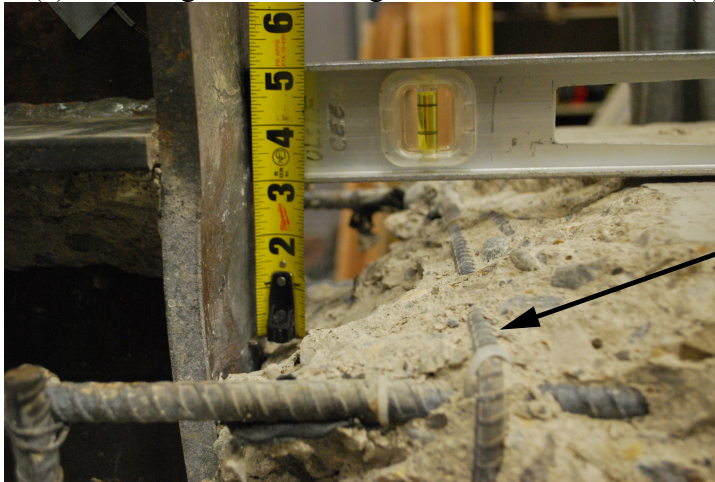
(e) Damage around flange
