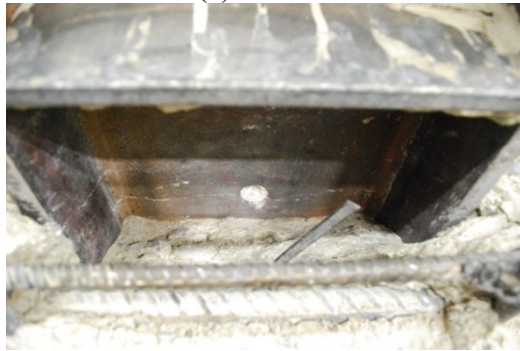
(c) Damage penetration
