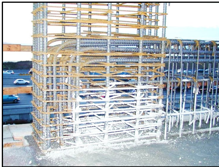
Figure 1.8 Steel congestion in an external beam-column joint caused by staggered hooked bars ( https://www.sefindia.org )
