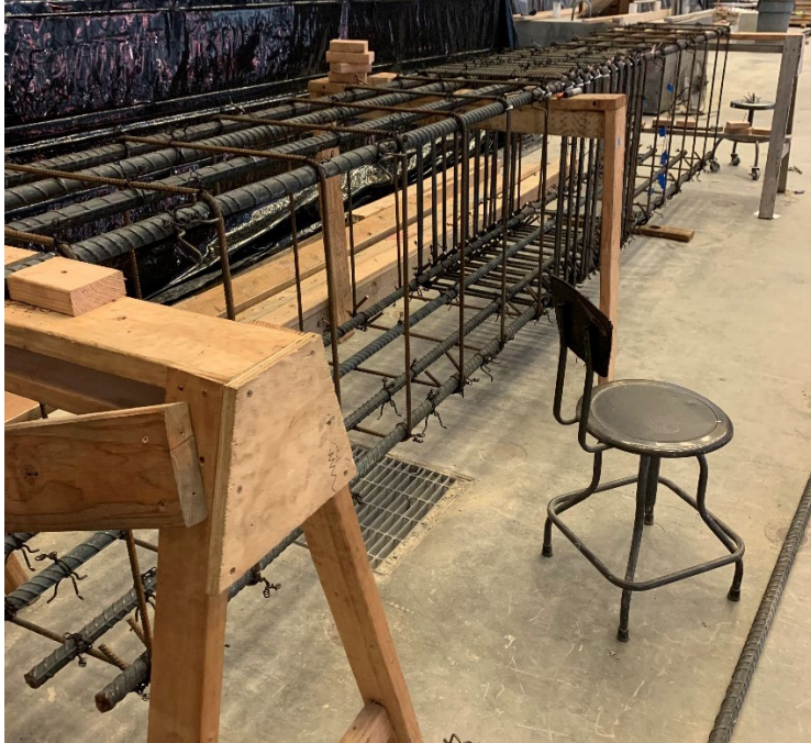
Figure 2.11 A typical reinforcement cage (steel cage)
