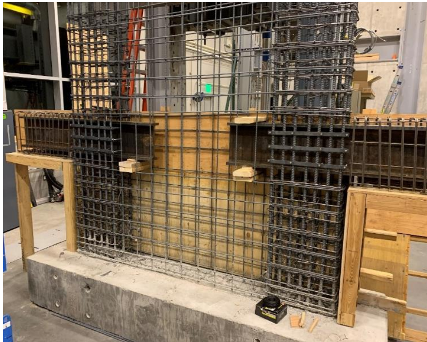
Figure 3.7. Photo of Reinforcement in Wall and Coupling Beams for SRC-W1 and SRC-W2
