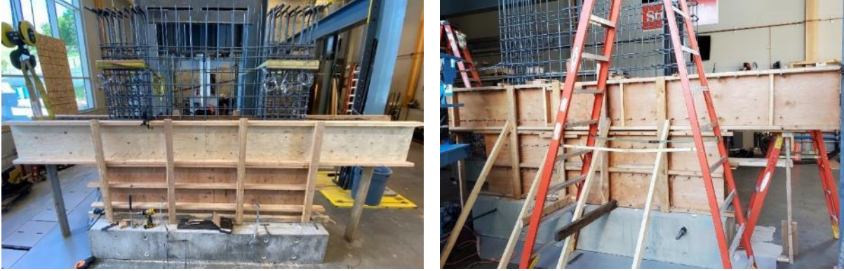
Figure 3.10. Photos Prior to Casting Concrete from Base of Wall to Top of Coupling Beams (Left Photo: SRC-W1 and SRC-W2. Right Photo: SRC-W3 and SRC-W4.)
