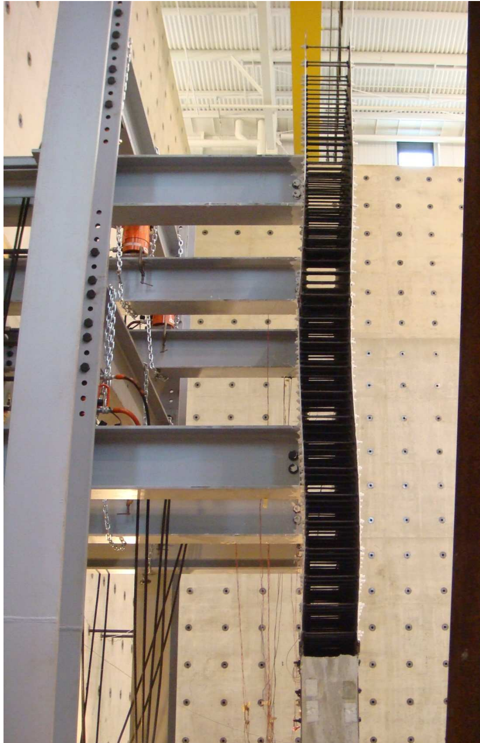
Figure 3.32 Distorted stability specimen at maximum applied load (168 kips) – View 1
