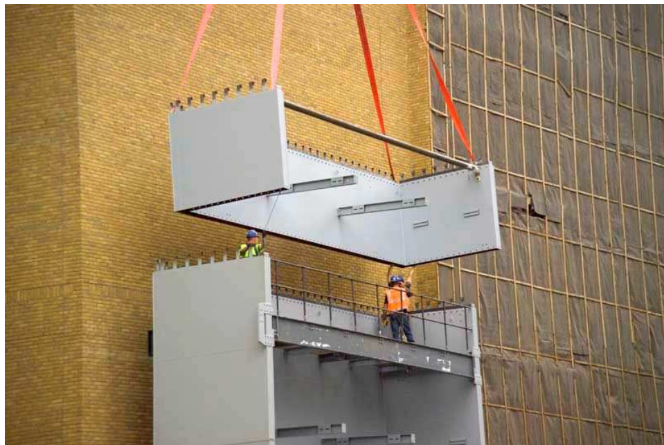
Figure 1.5 Lowering a Bi-Steel plate assembly unit in the field (from brochures by Corus)
