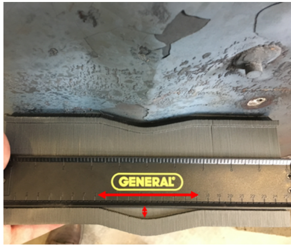
(d) Size of local buckling in CW1 with steel plate slenderness of 24
