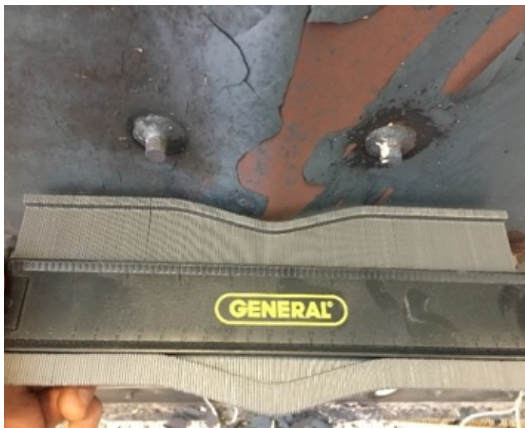
(c) Local buckling between tie bars
