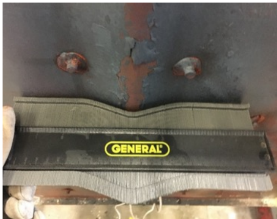
(c) Local buckling between tie bars
