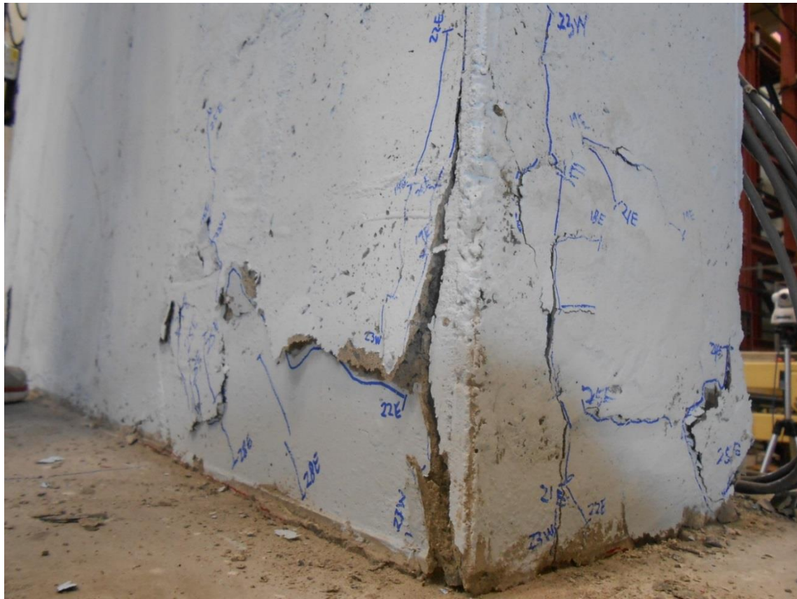
Figure 4-87 Photograph of observed concrete spalling at Cycle 28E on the West side Wall 3
