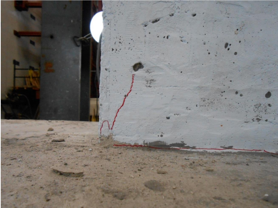
Figure 4-78 Photograph of observed splitting crack at Cycle 16W on the West side Wall 3
