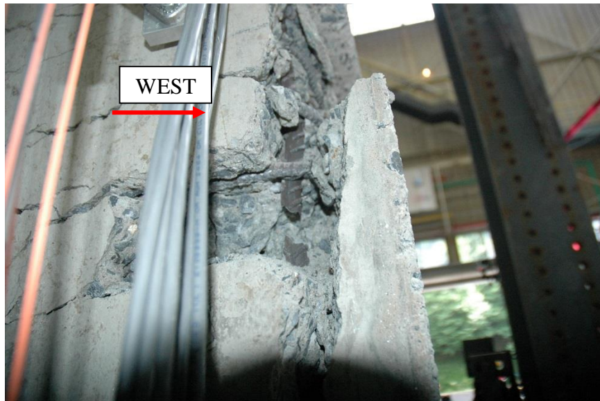
Figure 4-63 Photographs of observed fracture of longitudinal steel reinforcement at Cycle 39E Wall 2
