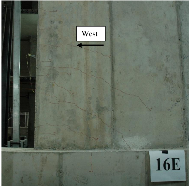
Figure 4-50 Photograph of observed initiation of concrete cracking on the West side Wall 2
