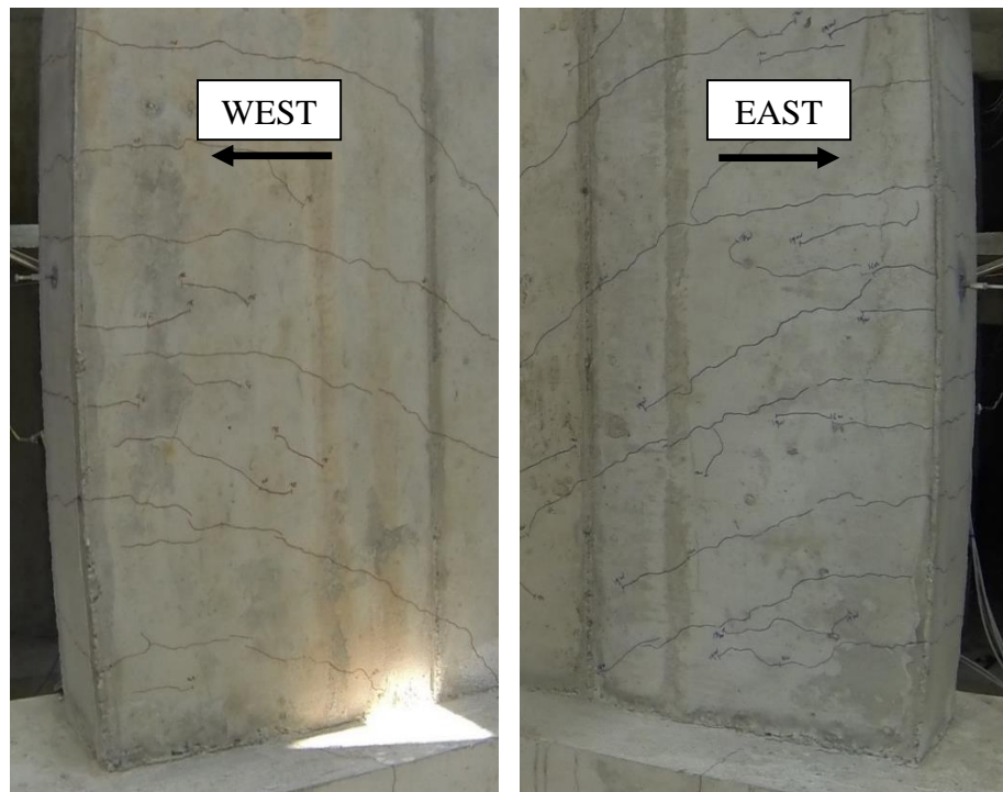
Figure 4-54 Photographs of observed wall conditions at the end of Cycle 19E Wall 2
