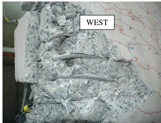
Figure 4-62 Photograph of observed buckling of longitudinal steel reinforcement at Cycle 39W Wall 2
