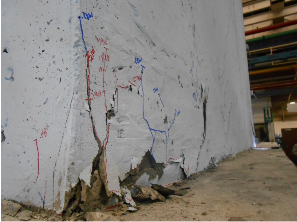
Figure 4-86 Photograph of observed concrete spalling at Cycle 28W on the West side Wall 3
