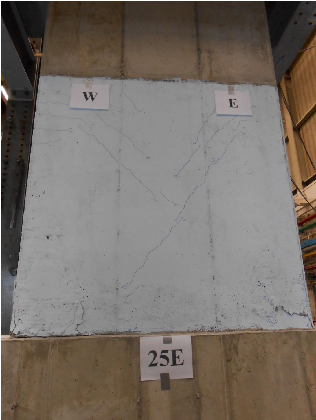
Figure 4-83 Photographs of observed diagonal cracks at Cycle 25E on the West side Wall 3
