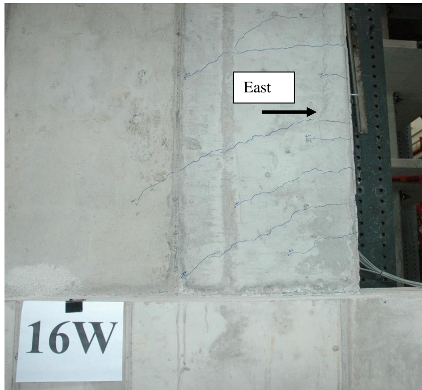
Figure 4-49 Photograph of observed initiation of concrete cracking on the East side Wall 2
