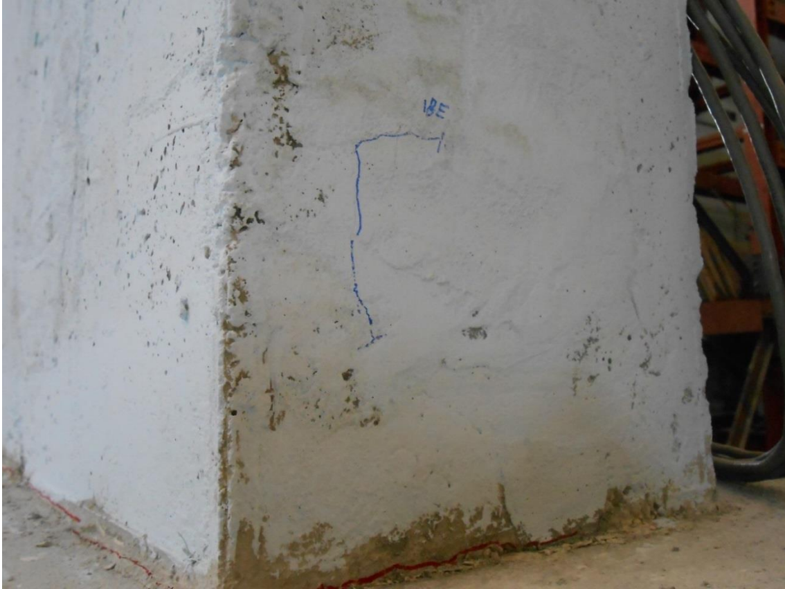
Figure 4-79 Photograph of observed splitting crack at Cycle 18E on the East side Wall 3
