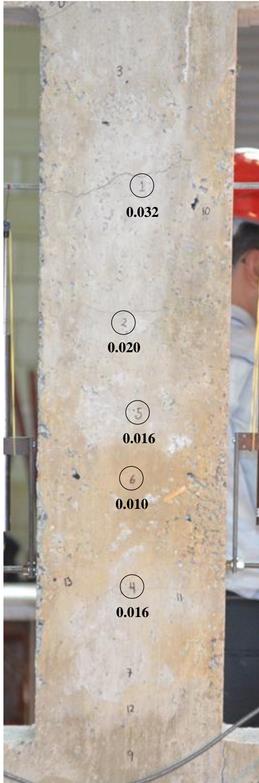
Figure 4-96: Cracks on east face of TS02 at Load Step 19
