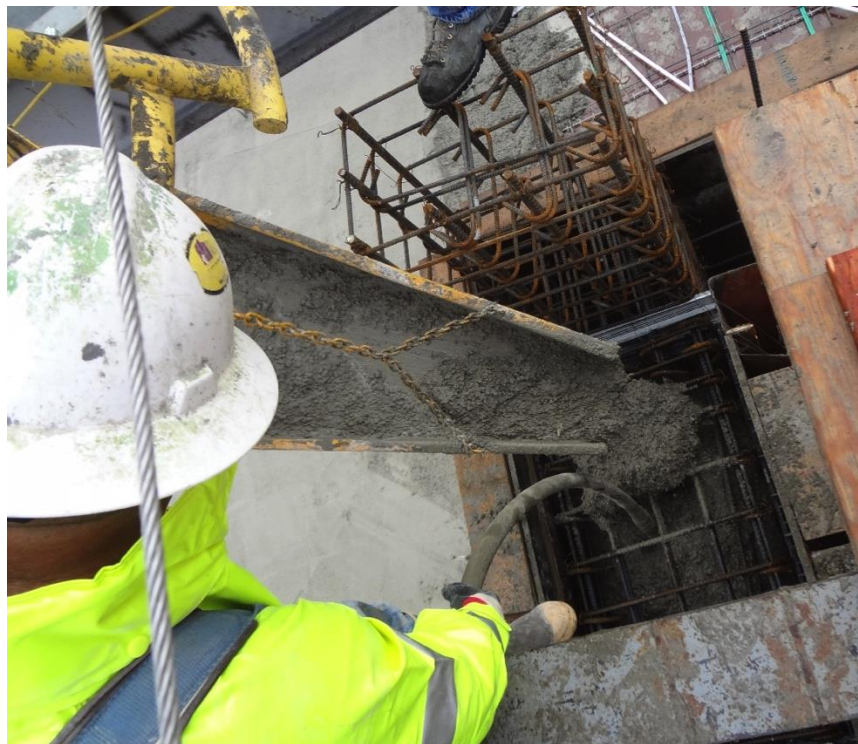
Figure 1.2: Casting of Fiber Reinforced Concrete Coupling Beam in The Martin Building, Seattle, WA
