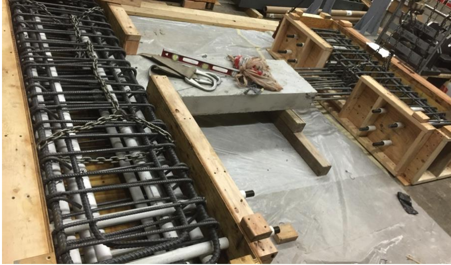
Figure 2.9: Precast FRC Coupling Beam Being Inserted Into End Block Reinforcement and Forms
