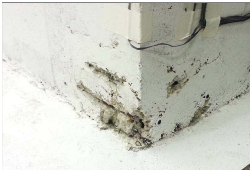
Figure 2.11: Voids in Wall 8 boundary element corner before patchwork
