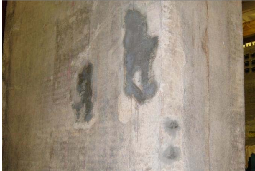
Figure 2.10: Wall 7 after patchwork near mid-height of web
