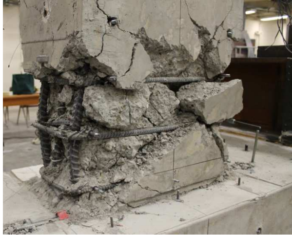
Figure 3.3.2: Failure Mechanism of SBH100 by Buckling of Longitudinal Bars Over Several Hoop Spacings
