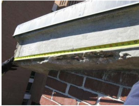
Figure 9-13. Overview of large spall at south end of curved concrete beam.
