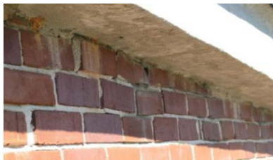
Figure 9-7. Poor installation of brick courses in curved portion of east elevation of High Bay
