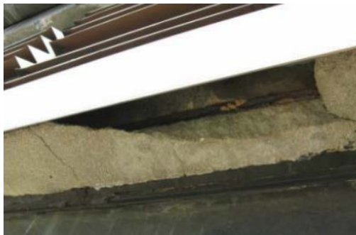
Figure 9-11. Exposed rebar that is now corroded because of material failure.
