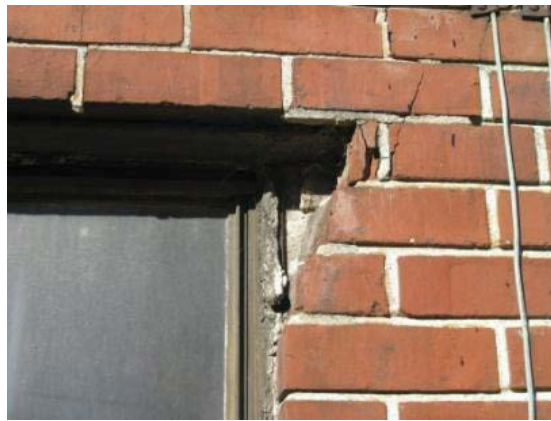
Figure 9-17. Damaged spalling brick at the end of a lintel.
