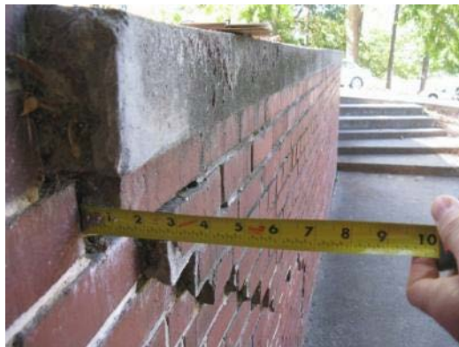
Figure 9-15. Displacement at the retaining wall.
