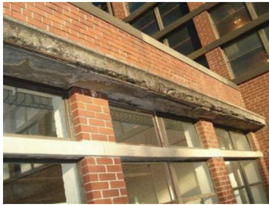
Figure 9-19. Spalled areas at the East elevation of the South office wing.
