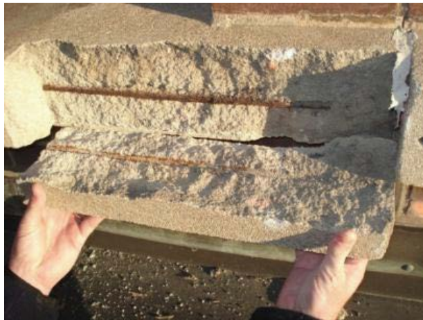
Figure 9-18. Spalled concrete sill.
