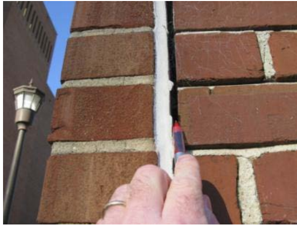
Figure 9-16. Failed expansion joint.
