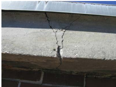
Figure 9-12. Transverse crack near midspan of curved concrete beam on east elevation of High Bay.
