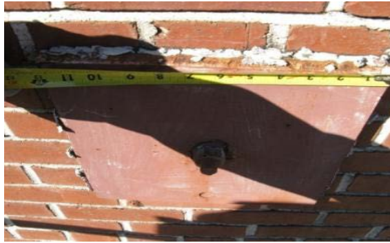
Figure 9-9. Failed sealants at anchor bolt and plate elevation of High Bay.
