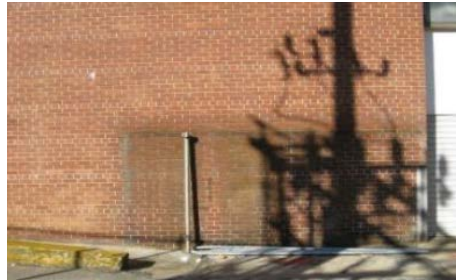
Figure 9-5. Stained area on east elevation of High Bay.
