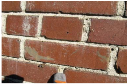
Figure 9-4. Typical deteriorated mortar joints on south elevation of High Bay.
