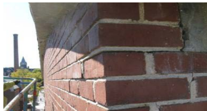
Figure 9-6. Crack and displaced brick masonry at north end of east elevation of High Bay.
